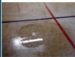
Playing surface Wet Floor or glass on floor
